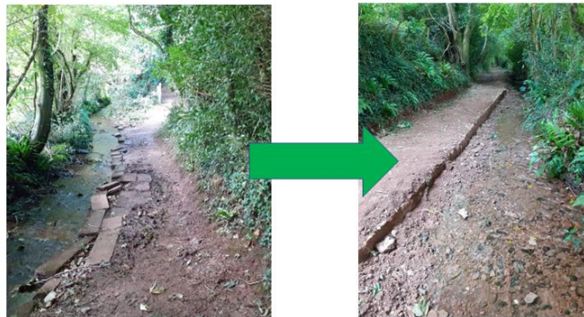
Figure 17 Watery Lane at Over Stowey before (left) and after (right) repairs made by the Scheme
